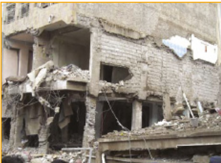
Image 26. Damaged building after an explosion.
