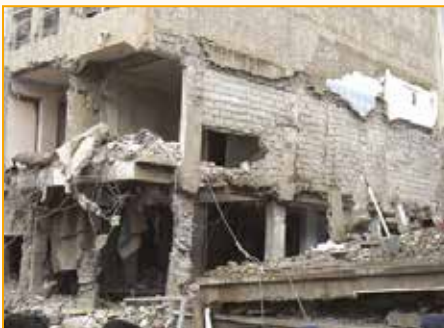
Obrazek 26. Damaged building after an explosion.
